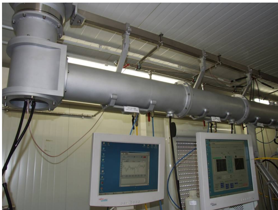
Figure 4: Main aerosol duct in container 4.
