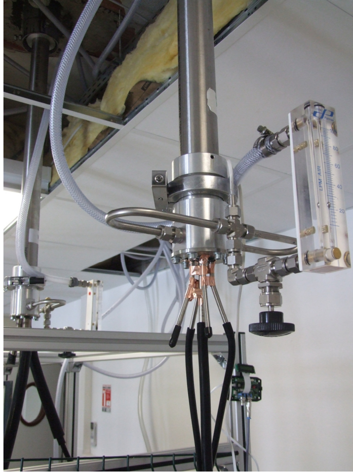
Figure 4: Aerosol splitter in the laboratory building.
